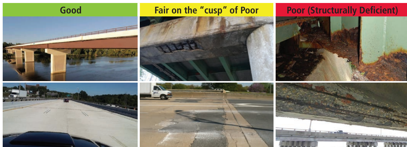
FIGURE 21 Examples of Good, Fair, and Poor-Rated Structures
