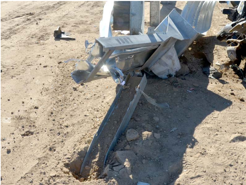
FIGURE 38. Test Article Damage
